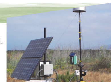
Solar Powered Gas Collection and Control System at Box Canyon
